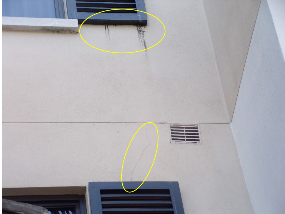
View of cracking stucco and staining from windowsill.
