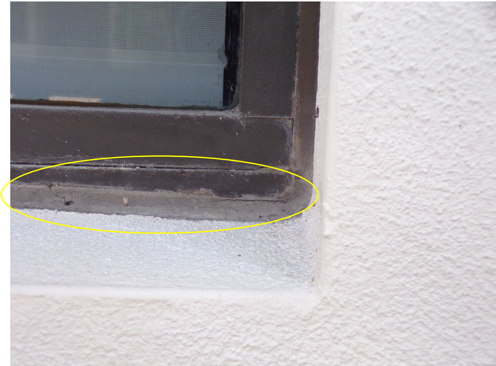
View of failing window sealant.
