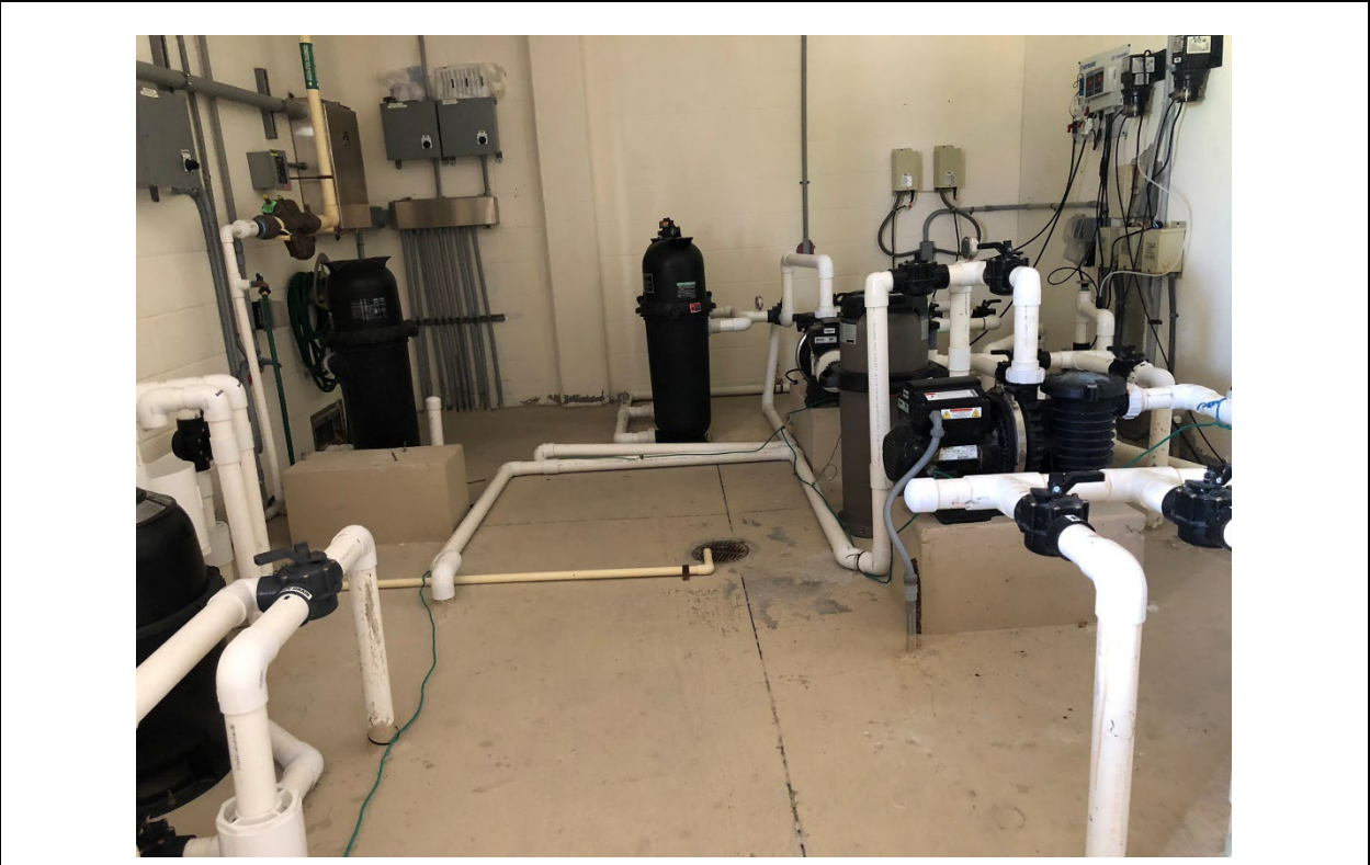
Overall view of pool equipment room.
