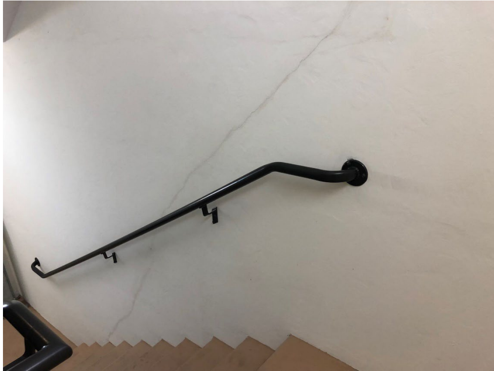
View of concrete cracking inside stairwell.
