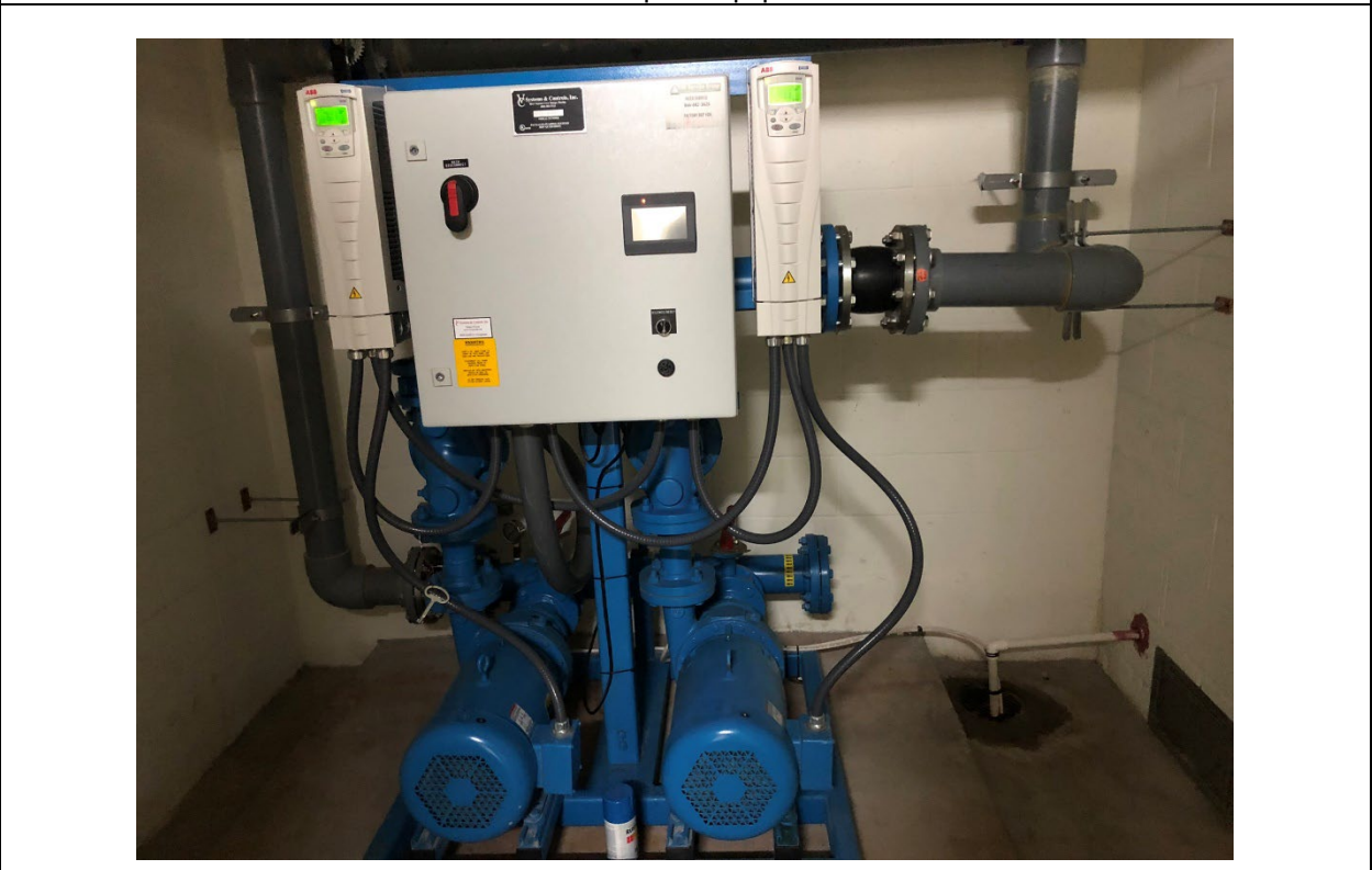
Overall view of domestic water pumps.
